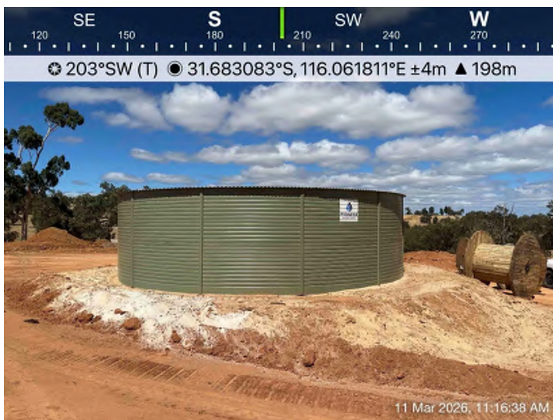
Plate 3: Compliant 100 kL fire water tank within Esme Crescent road reserve (facing south)
