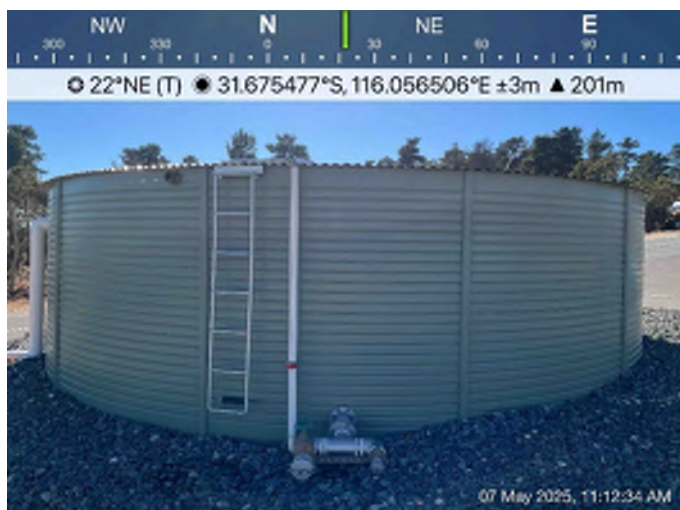
Plate 3: Compliant 100 kL fire water tank within Yarrimbah Drive road reserve (facing northeast)
