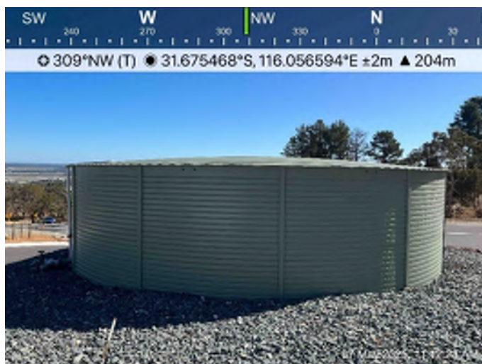
Plate 2: Compliant 100 kL fire water tank within Yarrimbah Drive road reserve (facing northwest)
